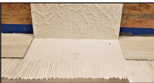
To verify proper coverage and embedment, lift a tile and examine the back of the tile for mortar coverage, and examine the substrate for ridge collapse. This photo is an example of ideal coverage and embedment.
